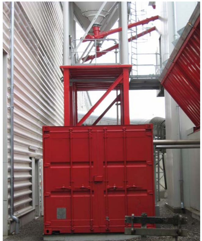
fig 2. TURBOMATIC thermal energy unit at Dachser gmbH & Co. KG
