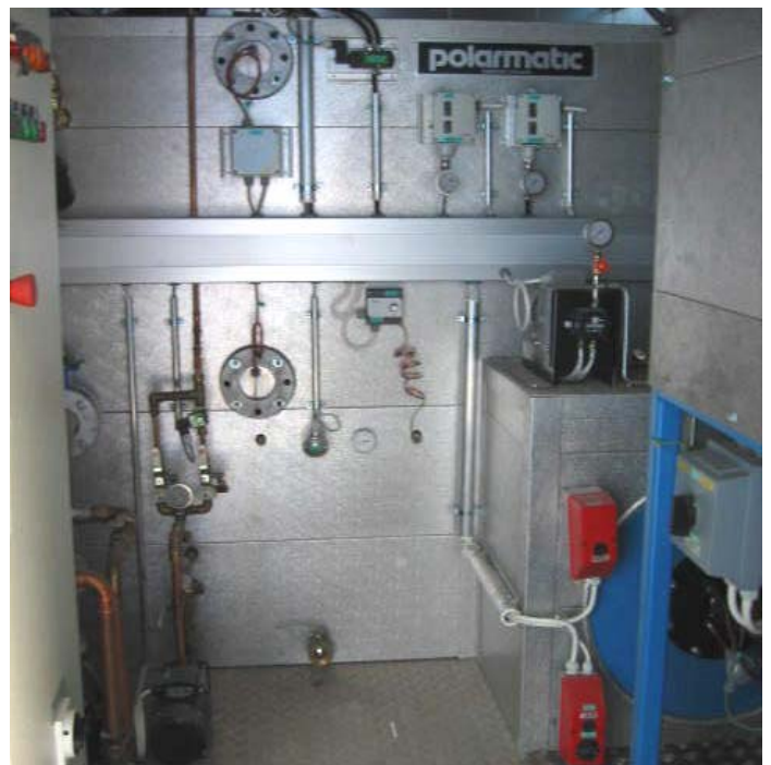
interior view of the Turbomatic thermal energy unit
